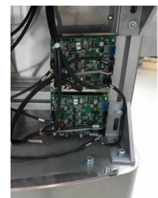
Right side boards: B1 (bottom) and B2 circuits
